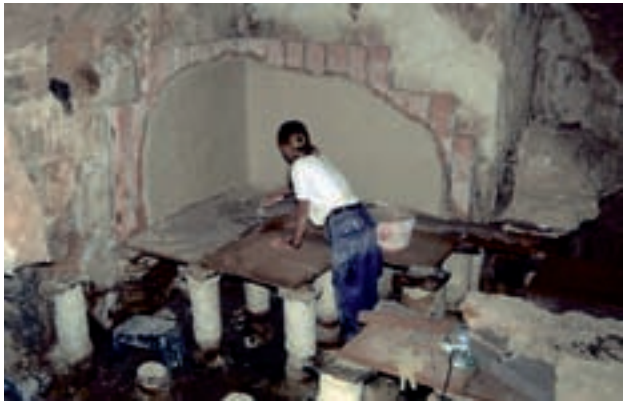
Fig. 1 The Large Baths, Masada, Israel. A model of the suspended floor and of the hot air circulation system on the walls, during restoration in the caldarium .
